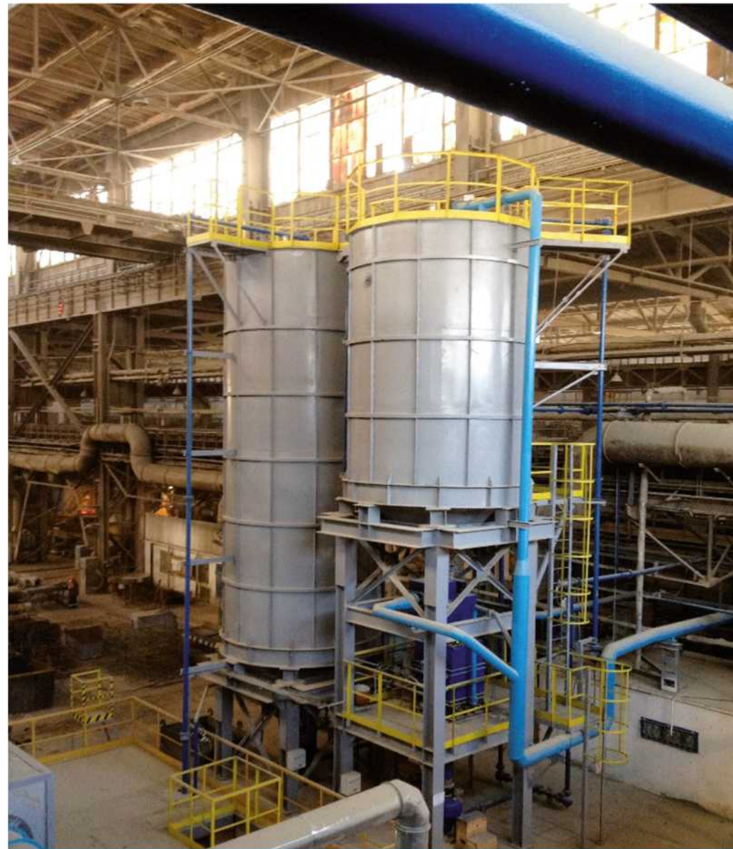
Fresh sand and reclaim bin
